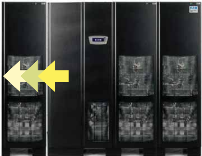
On site upgrade 550 kVA redundant
