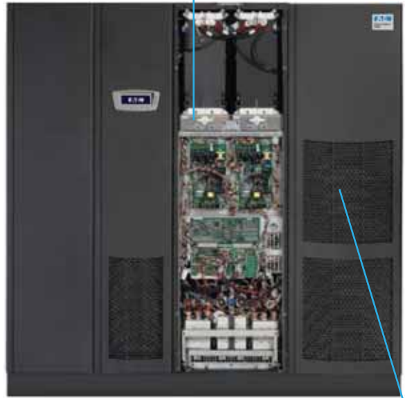
Concurrent maintenance in Power Xpert™ 9395 550 kVA ...while this module carries the load
